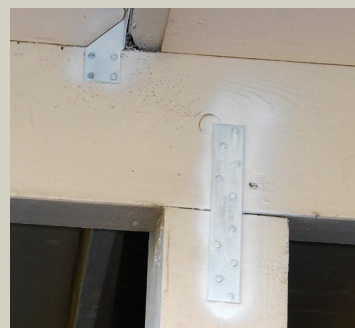
Figure 4-26. In this retrofit example, a hurricane clip attaches the roof structure to a horizontal ridge beam, which is in turn attached to the vertical post with a metal strap. This is an attempt to tie the load from the roof to the foundation, or create the complete load path connection. Note that these clips and straps are in the process of being painted. Source: Hurricane Protection Services.
